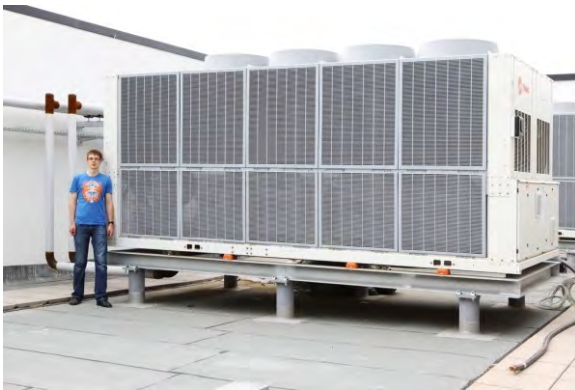
Fig. 5: One of two chillers on the roof
