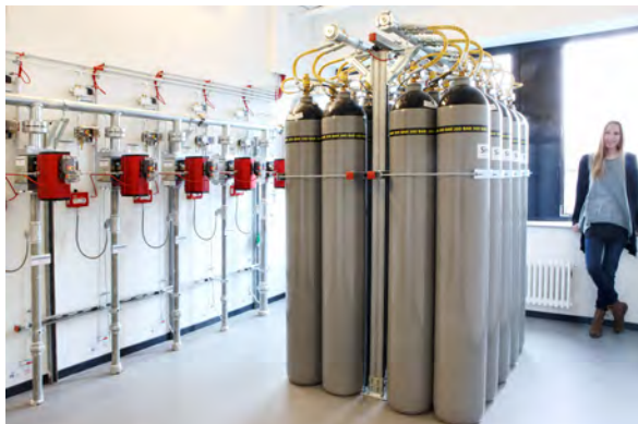
Fig. 8: Nitrogen fire suppression
