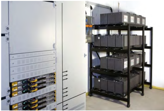
Fig. 3: One of two uninterruptible power supply units (UPS)
