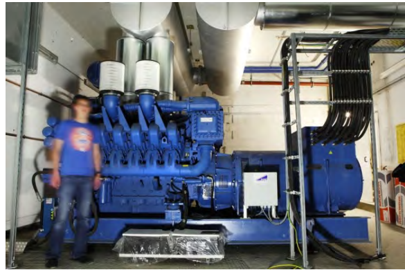
Fig. 4: The emergency power system (Diesel engine)
