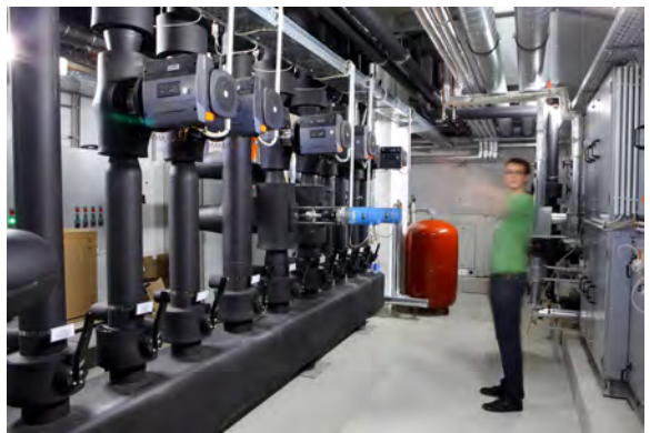
Fig. 6: Cooling and Heating central in the cellar
